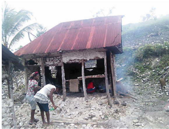
A hurricane-damaged home in the village of Gris-Gris. (Photo courtesy of St. Rose of Lima parish)
